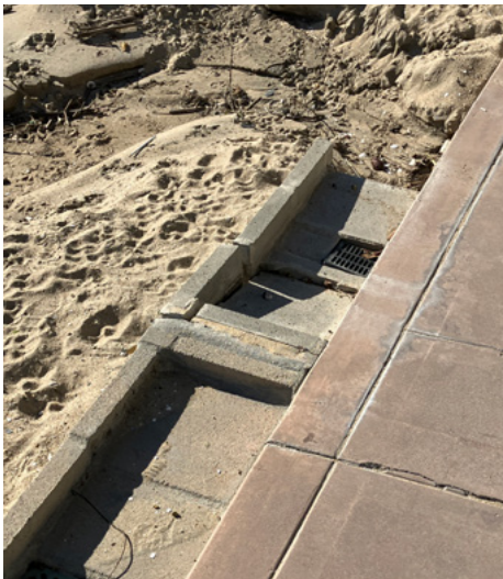
Failed beach drain
