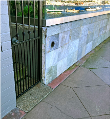
Lot that drains onto the sidewalk
